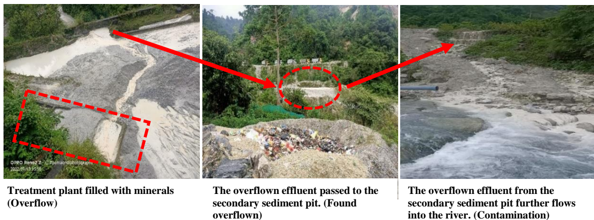
Picture 5: Sludges overflowing from the treatment plant to the Chunaikhola River below.
