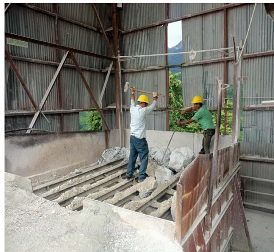
Picture 1: Regular workers without proper PPE (safety gloves, protective goggles, reflective jackets and ear plugs etc.)
